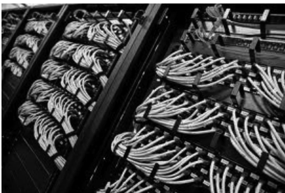
FIGURE 10.2 Networking infrastructure in data centers.
